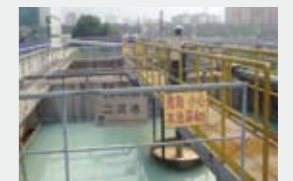
Chemical treatment COD removal facilities
