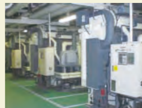
Upgraded absorption refrigeration units
