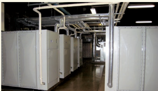
Thermal storage heat pump system
