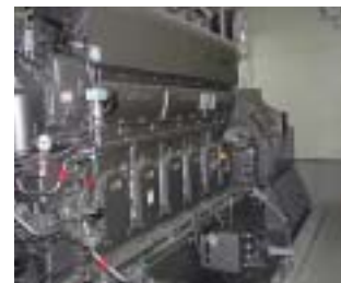
Cogeneration Equipment at Citizen Machinery
