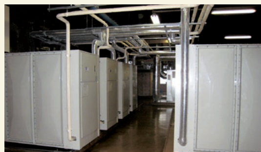
Thermal storage heat pump system
