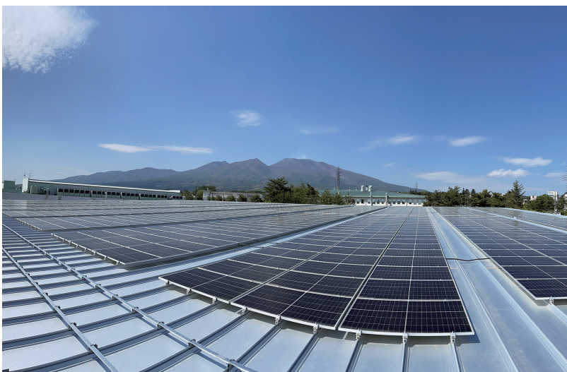
Solar panels installed at the Karuizawa Headquarters factory of the Machine Tool business (Citizen Machinery)
